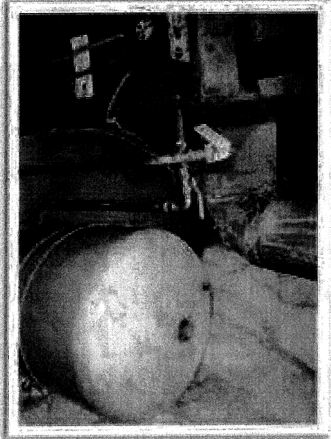
MECHANICALS IN BOILER ROOM
